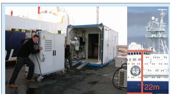
Fig. 1: (left) Mounting the lidar within the OCEANET-container at the pier of Punta Arenas. (right) The OCEANET-container was deployed at the upperdeck, starboard of the research vessel Polarstern .
