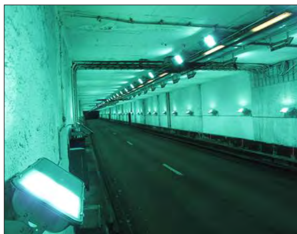
Fig. 3: Test section Leopold II tunnel, Brussels with the applied photocatalytic concrete and 236 additional UV-light sources. (Photo: PhotoPAq consortium)
